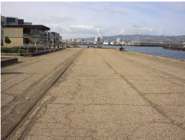
Pier at southeastern end of Wind River site (north of Trail Section 3, Sheet 6).
