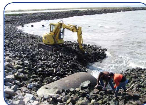
The City has conducted a series of engineering studies to determine the best ways to protect neighborhoods during big storms and sea level rise.
