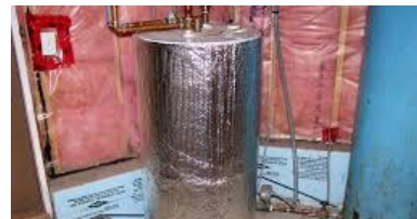
Water Heater Blanket
