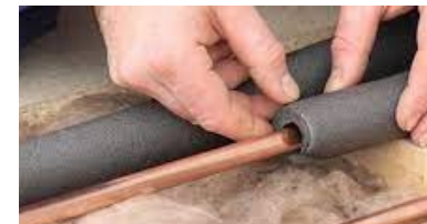
Hot Water Pipe Insulation
