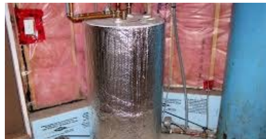
Water Heater Blanket
