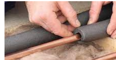
Hot Water Pipe Insulation
