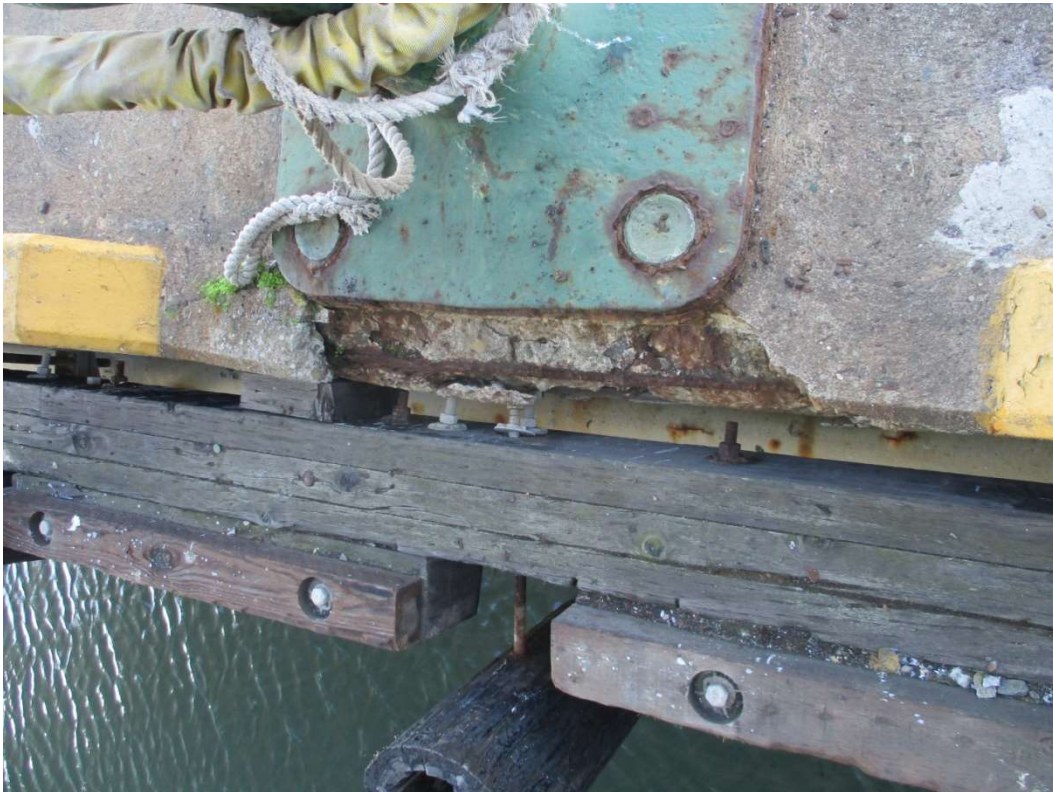
Photo 26 – Corrosion spalling of concrete at mooring hardware at Pier 3
