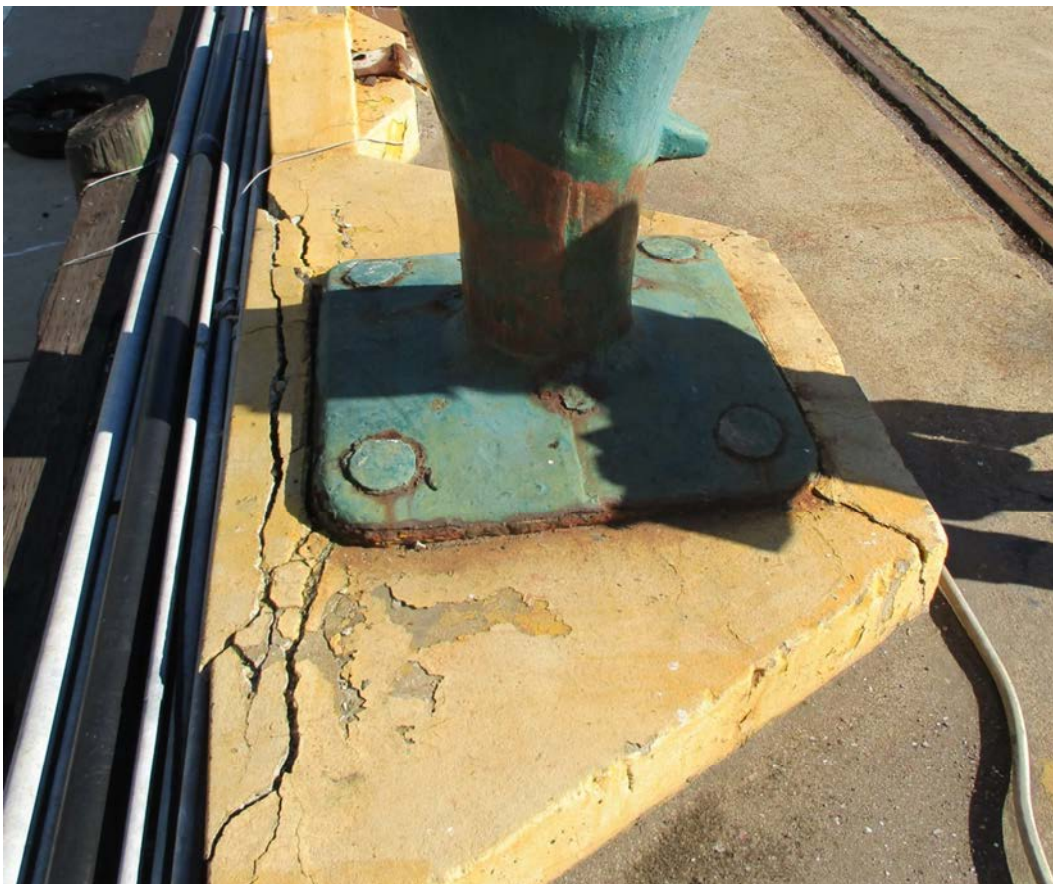
Photo 18 – Spalling in front of mooring bollard base at Pier 2
