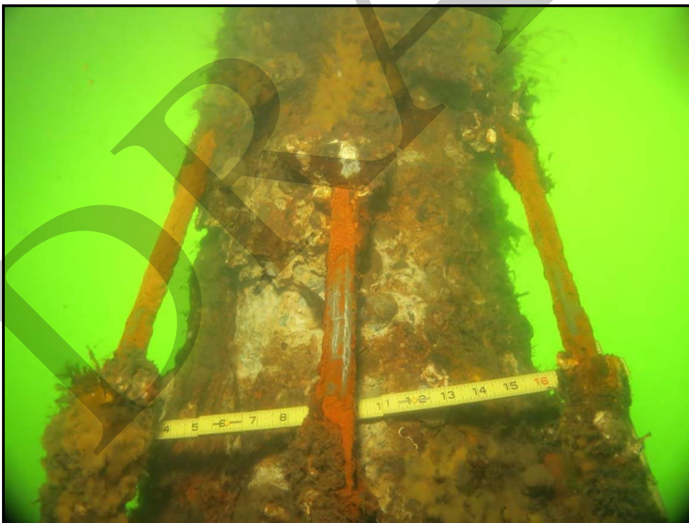
Photo 20: Severe loss of concrete section due to chemical deterioration with exposed reinforcing.
