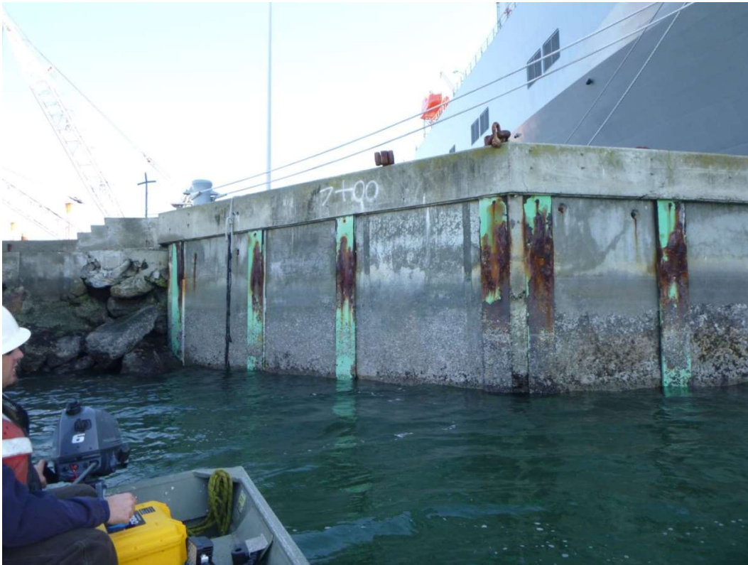
Photo 2 - Typical condition of concrete panels at Pier 1
