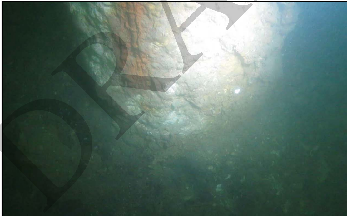
Photo 16: Pier 2, Pile 43-H - Exposed reinforcing near the mudline.
