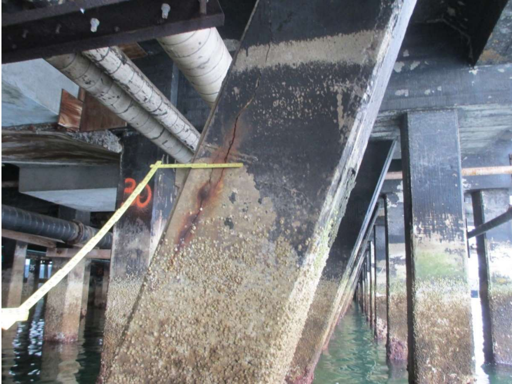
Photo 13 – Pile rated Major due to corrosion spalling at Pier 2
