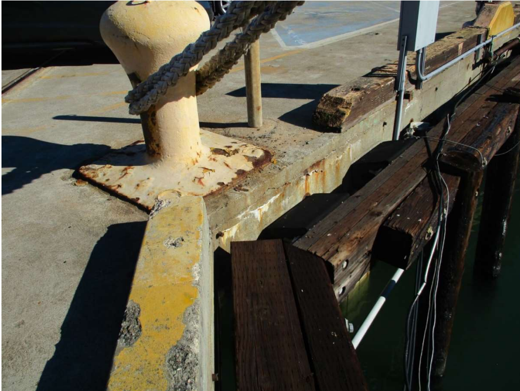
Photo 25 – Typical condition of mooring hardware at Pier 3
