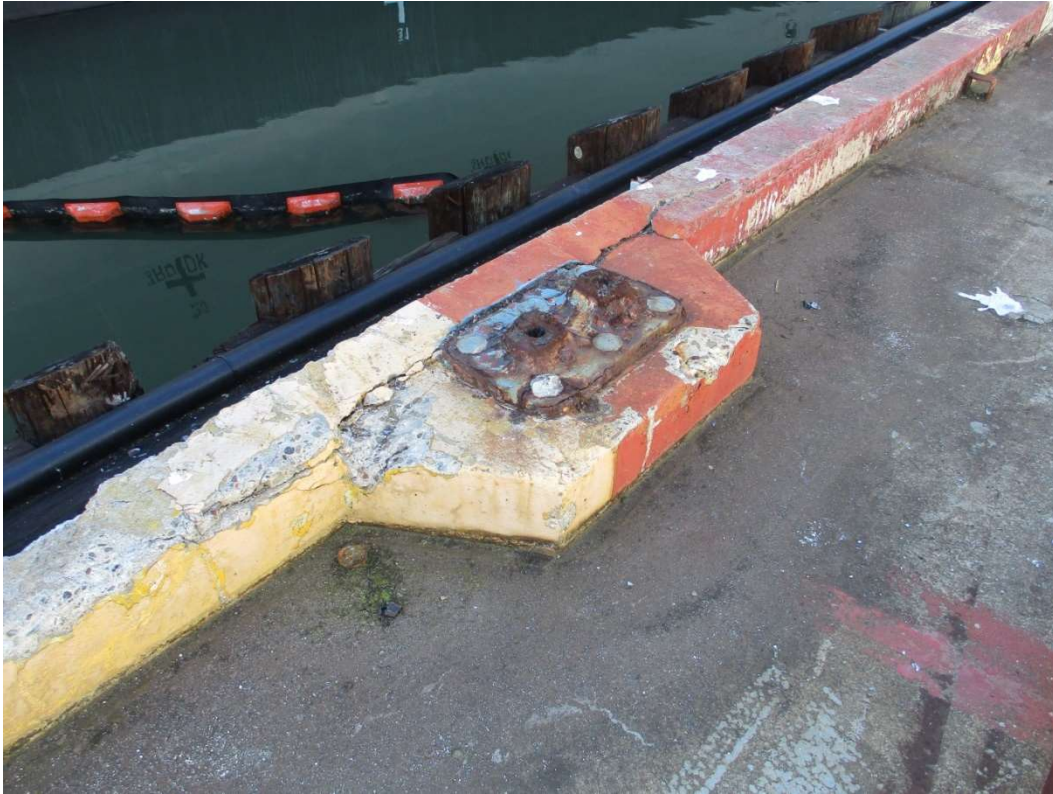
Photo 17 – Broken cleat at Pier 2
