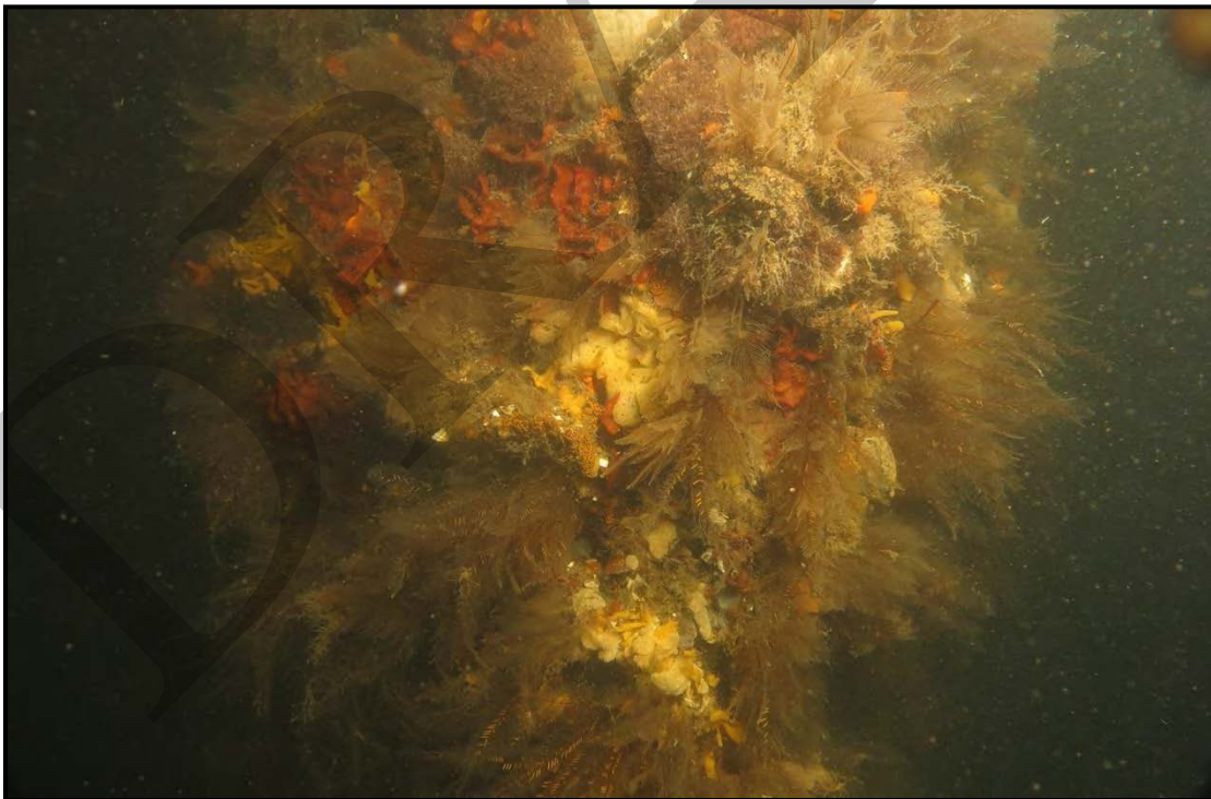
Photo 4: Typical marine growth on structural piles.
