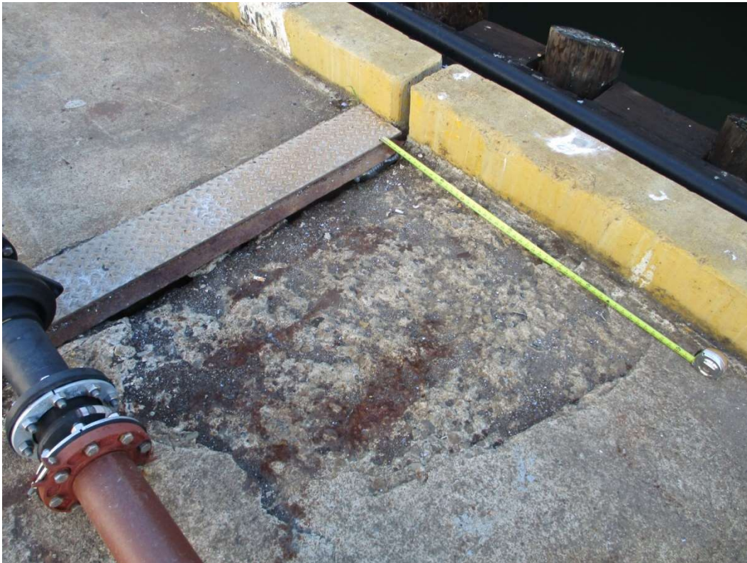
Photo 15 - Spalling of deck at expansion joint at Pier 2
