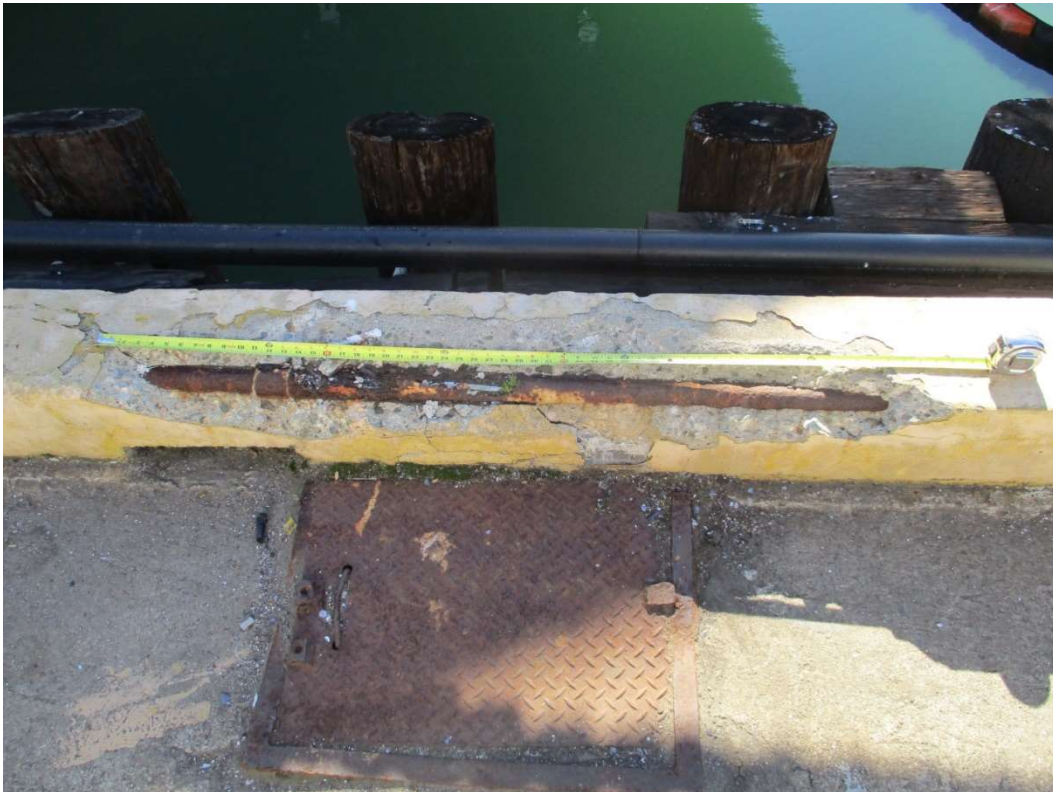
Photo 20 – Spalling of curb at Pier 2
