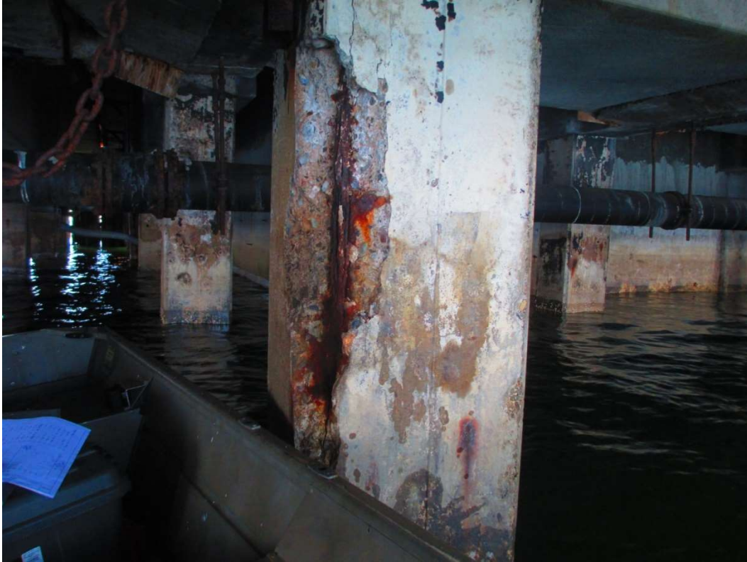
Photo 11 – Pile rated Severe due to corrosion spalling at Pier 2
