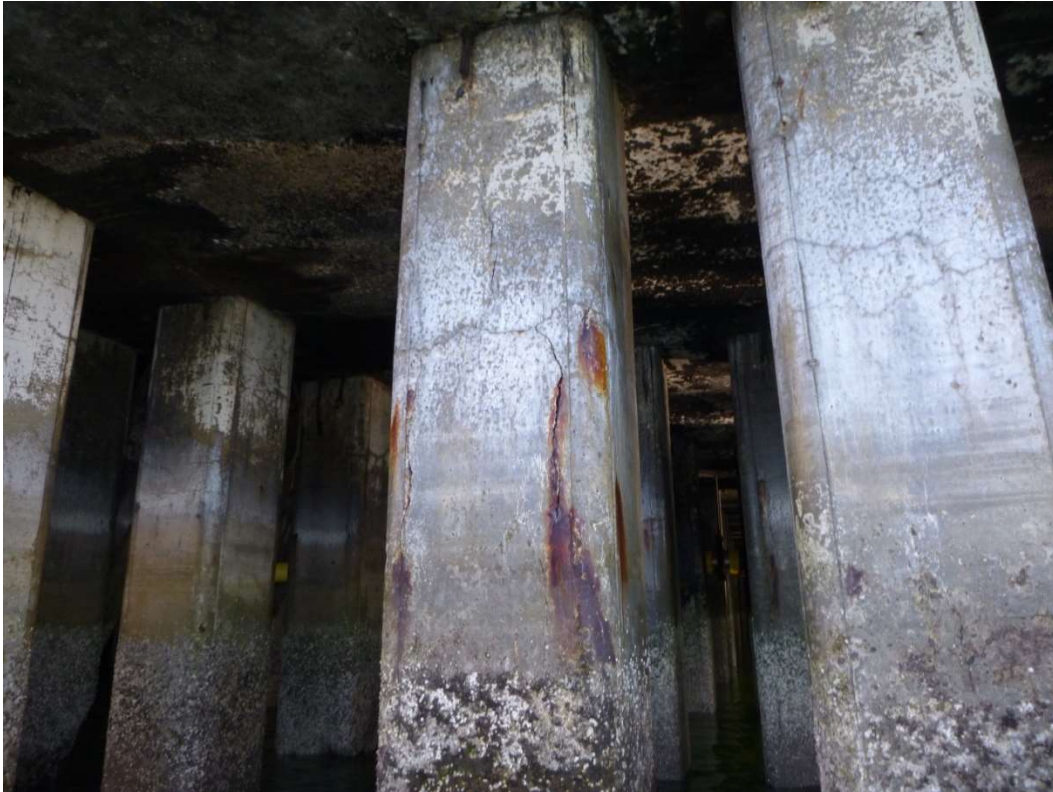
Photo 21 – Corrosion cracking of pile extension at Pier 3
