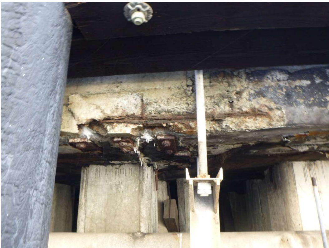
Photo 24 – Corrosion spalling of deck edge at Pier 3
