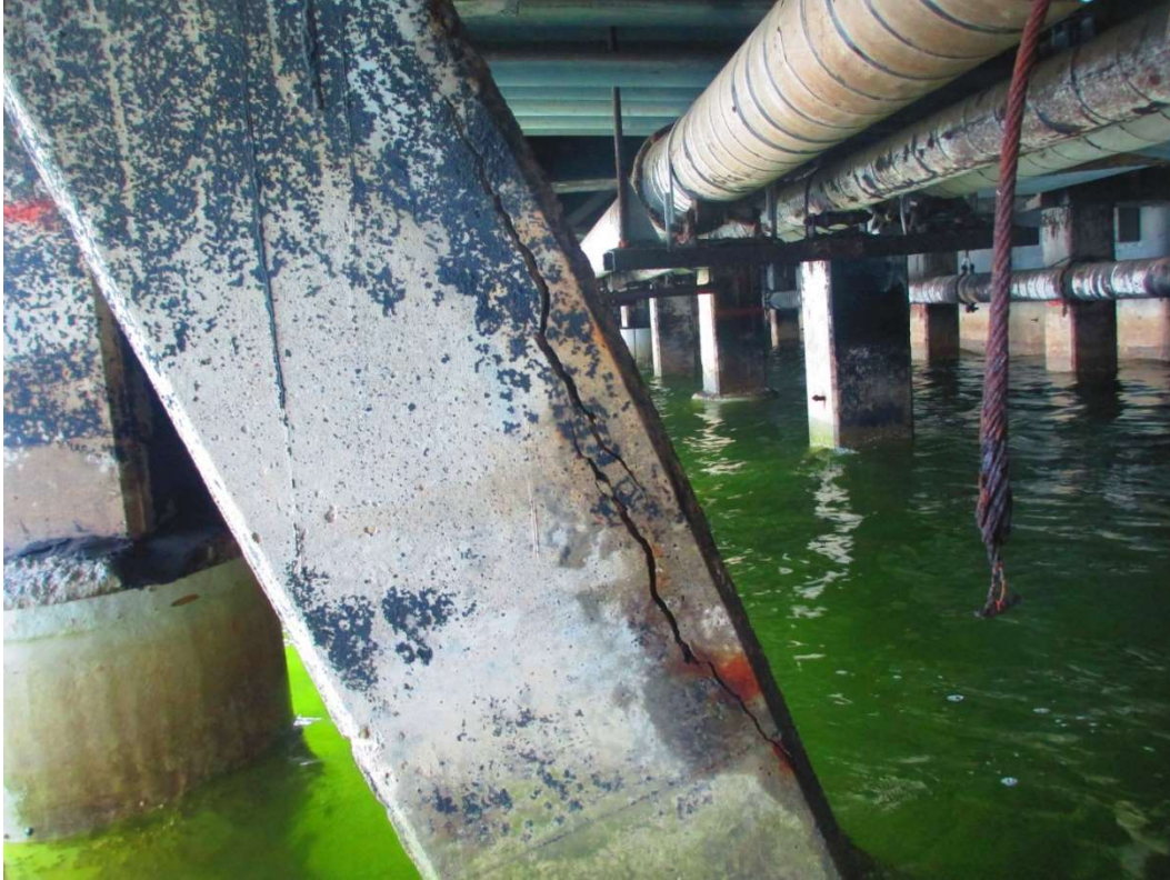
Photo 9 – Pile rated Major due to corrosion spalling at Pier 2
