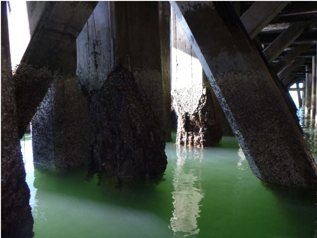
Photo 22 – Deterioration of lower part of pile extension at Pier 3
