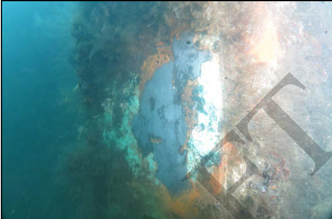
Photo 9: Coating loss and corrosion on steel king pile at Pier 1.
