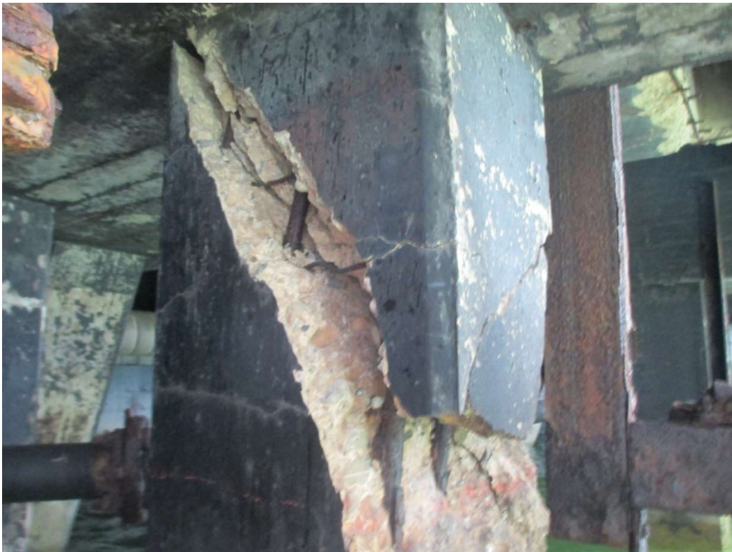
Photo 12 – Pile rated Severe due to impact damage at Pier 2
