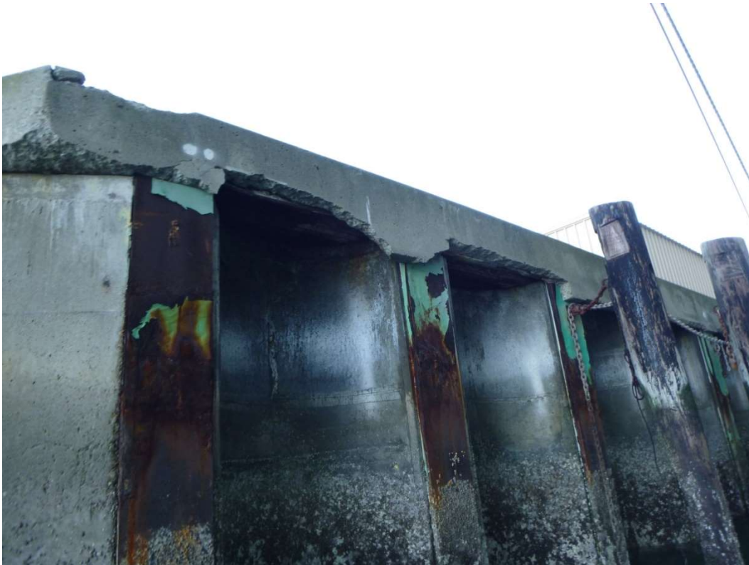
Photo 4 – Spalled lip of pile cap at Pier 1
