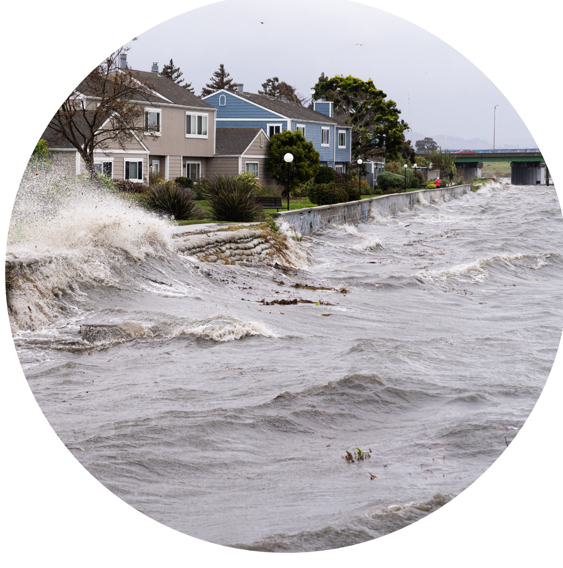
Wave overtopping at Elsie Roemer shoreline
