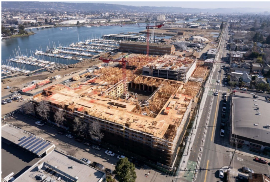
New multifamily rental housing coming online in 2022 at the Alameda Marina project on Clement Avenue.
