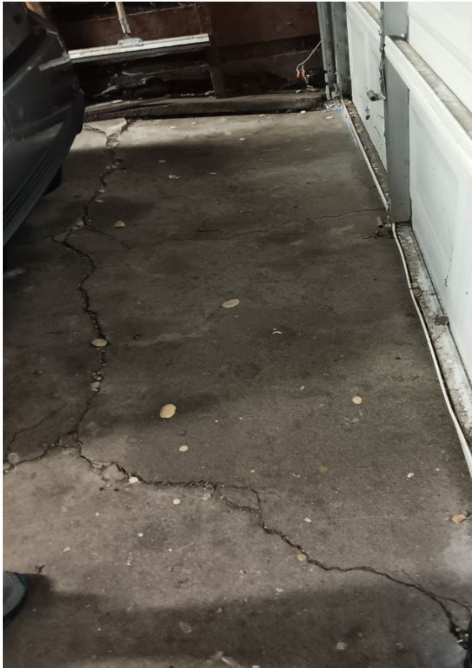
Photo 3. Cracking of structure foundation
