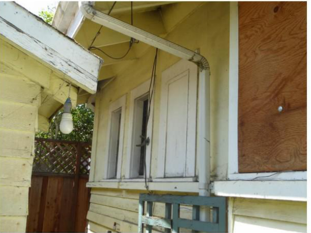
Figure 13: Missing casement windows on south end of east façade.
