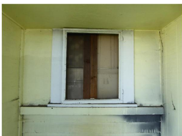
Figure 11: Missing window inside west porch recess.
