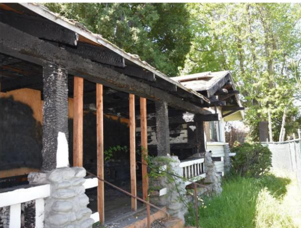
Figure 4: North façade with burn-damaged porch.
