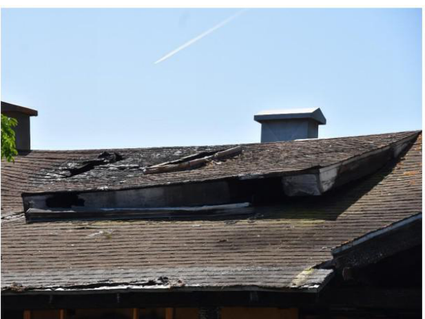
Figure 9: Collapsed shed roof dormer.
