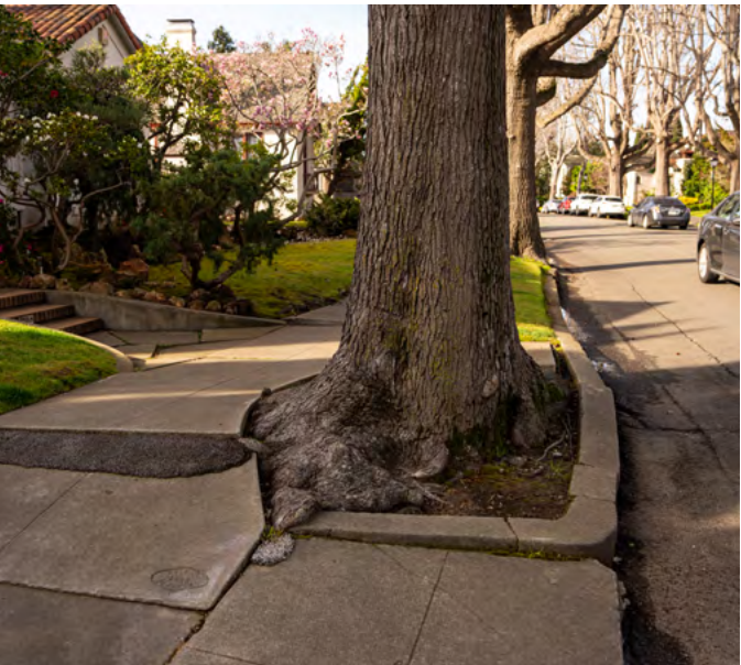
Photo 5: Displacement of sidewalk panels encroaching into the walkway at trunk of tree
