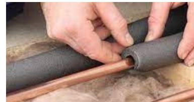
Hot Water Pipe Insulation
