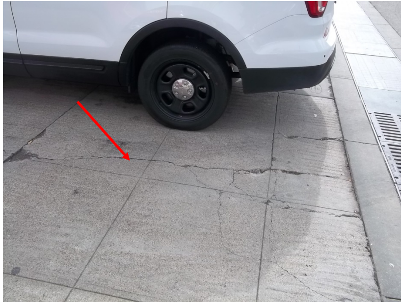
Photograph 5: Cracked pavement at south end of west driveway
