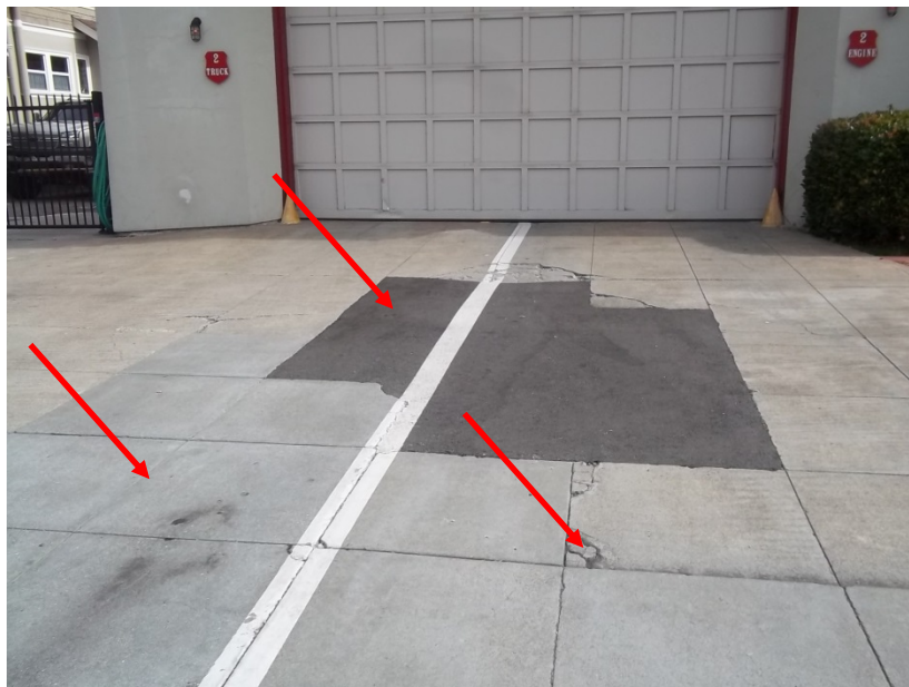
Photograph 2: South apparatus driveway looking north at newer concrete panels, asphalt concrete patch, and corner breaks in older panels
