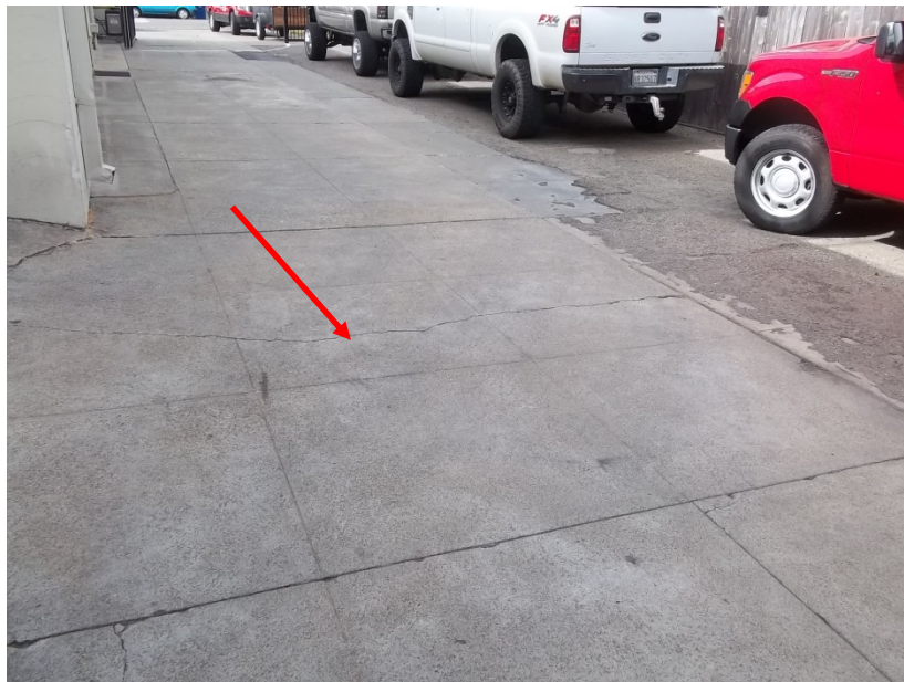
Photograph 6: Cracked pavement at north end of west driveway
