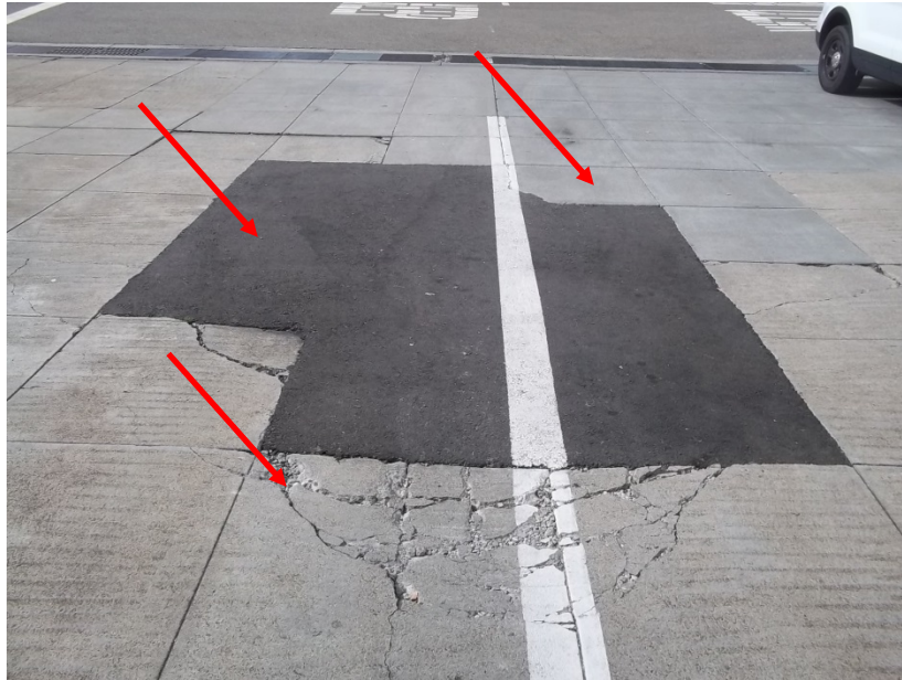
Photograph 3: South apparatus driveway looking south at newer concrete panels, asphalt concrete patch, and severe cracking in older panels
