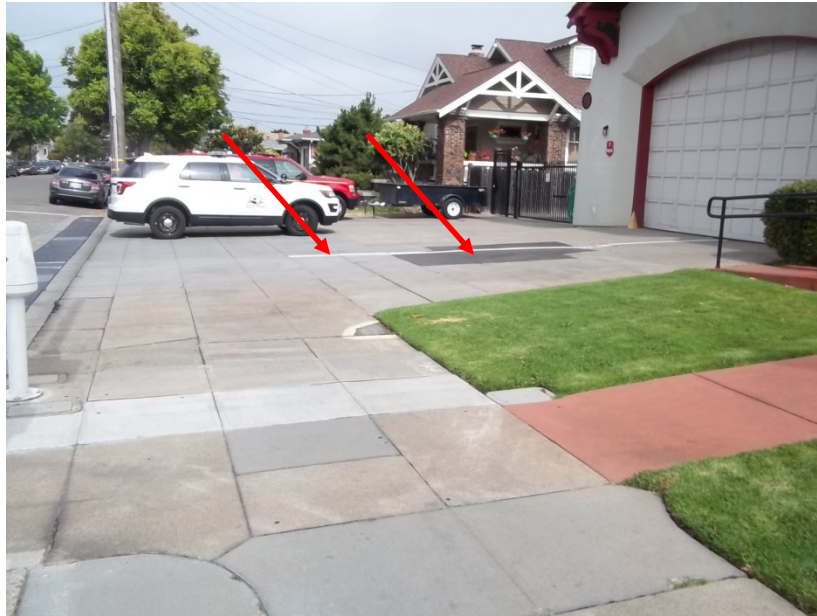
Photograph 1: South apparatus driveway looking west at newer concrete panels and asphalt concrete patch
