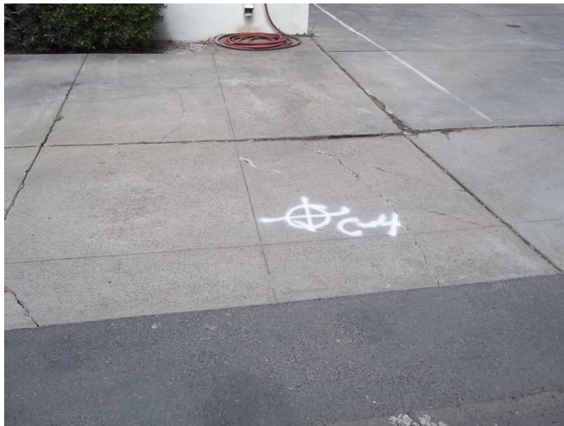
Photograph 10: Boring B-4 location in cracked panel on east driveway
