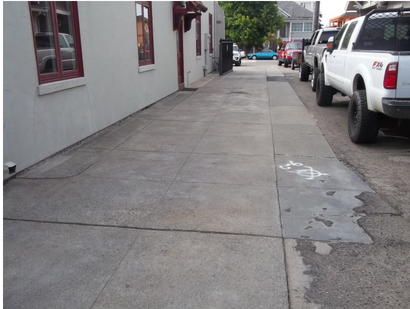
Photograph 9: Boring B-3 location near depressed area in west driveway
