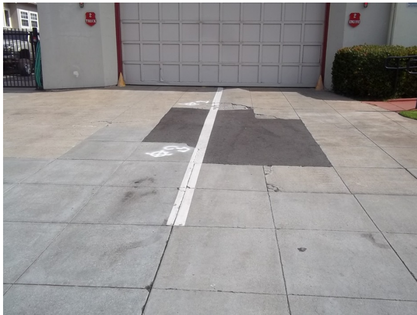
Photograph 8: Boring B-1 location in old concrete panel near asphalt patch on south apparatus driveway and Boring B-2 location in newer concrete panel near asphalt patch
