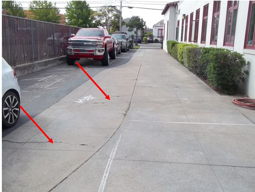
Photograph 7: Cracked pavement at east driveway
