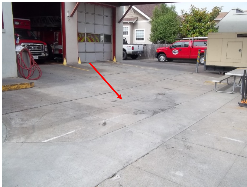
Photograph 4: Cracked concrete pavement north of central building
