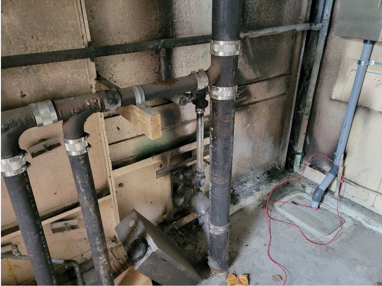
Figure 9 Harrington Utility Closet Plumbing 3
