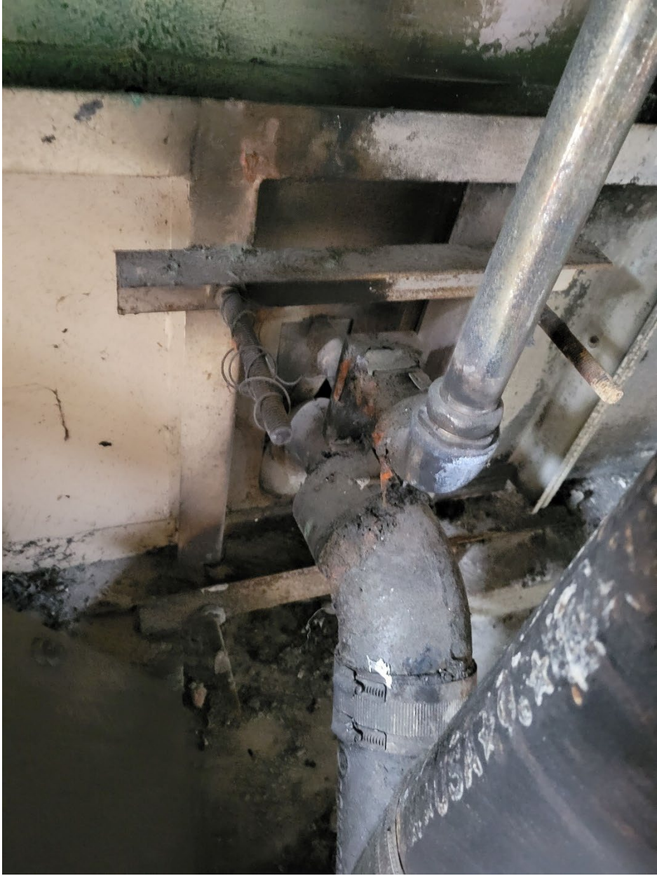
Figure 7 Harrington Utility Closet Plumbing 1
