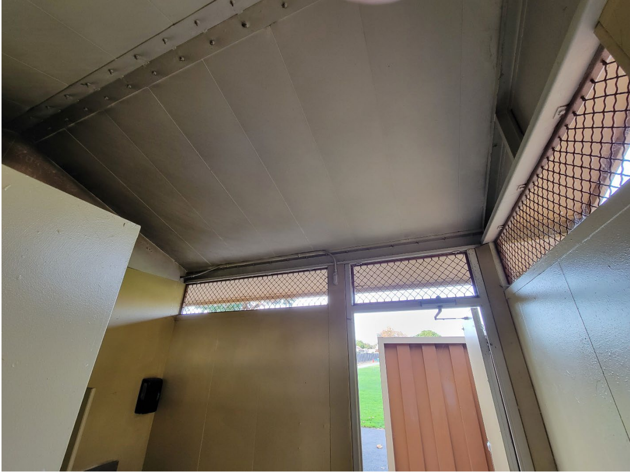
Figure 20 Harrington Men's Restroom Ceiling 2
