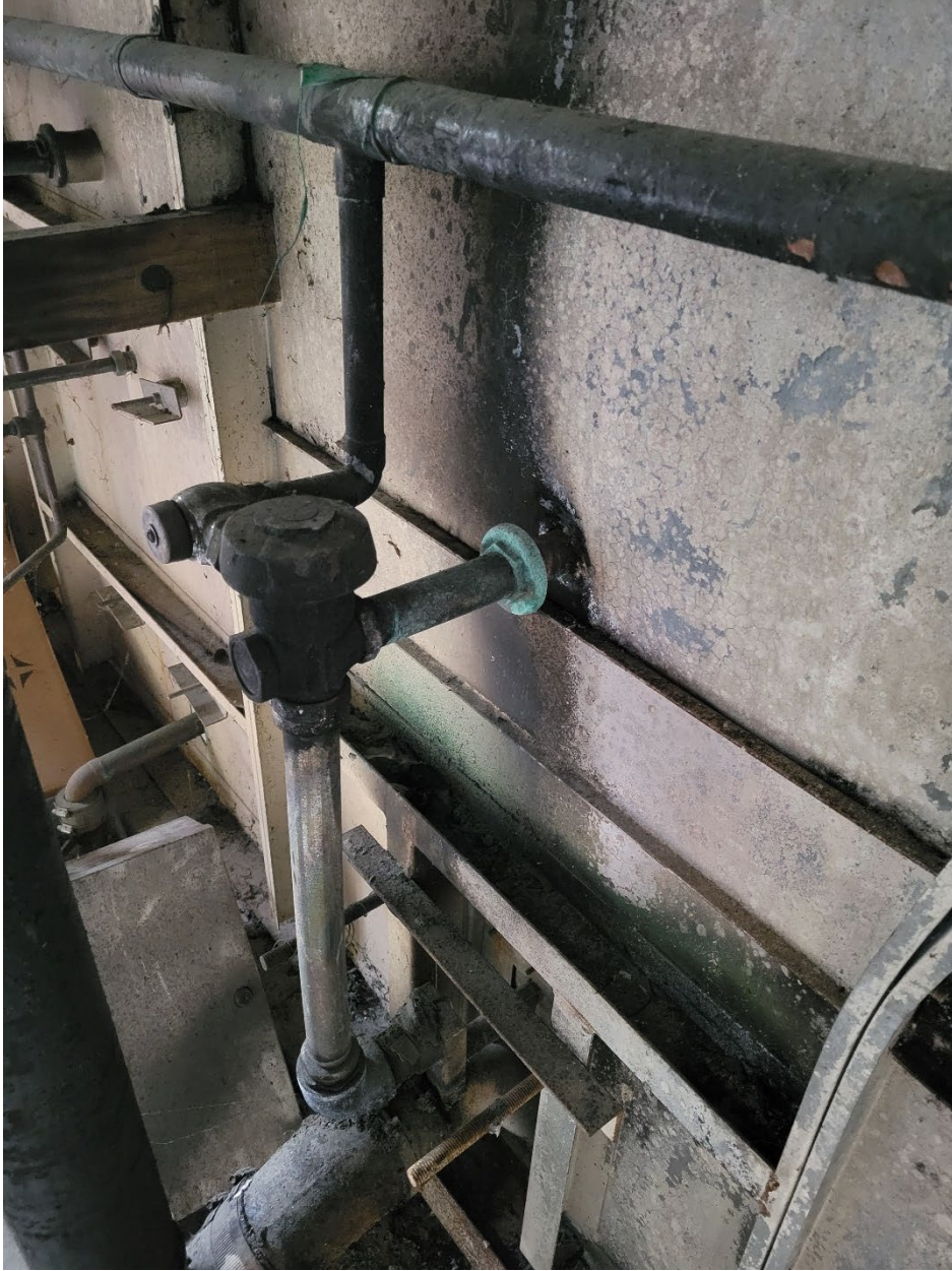
Figure 8 Harrington Utility Closet Plumbing 2
