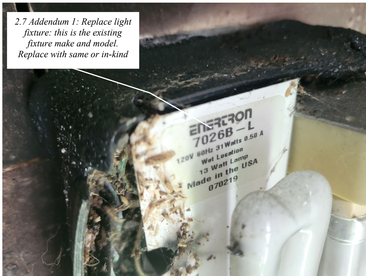
Figure 21 Addendum 1: Existing Restroom Light Fixture Model Information
