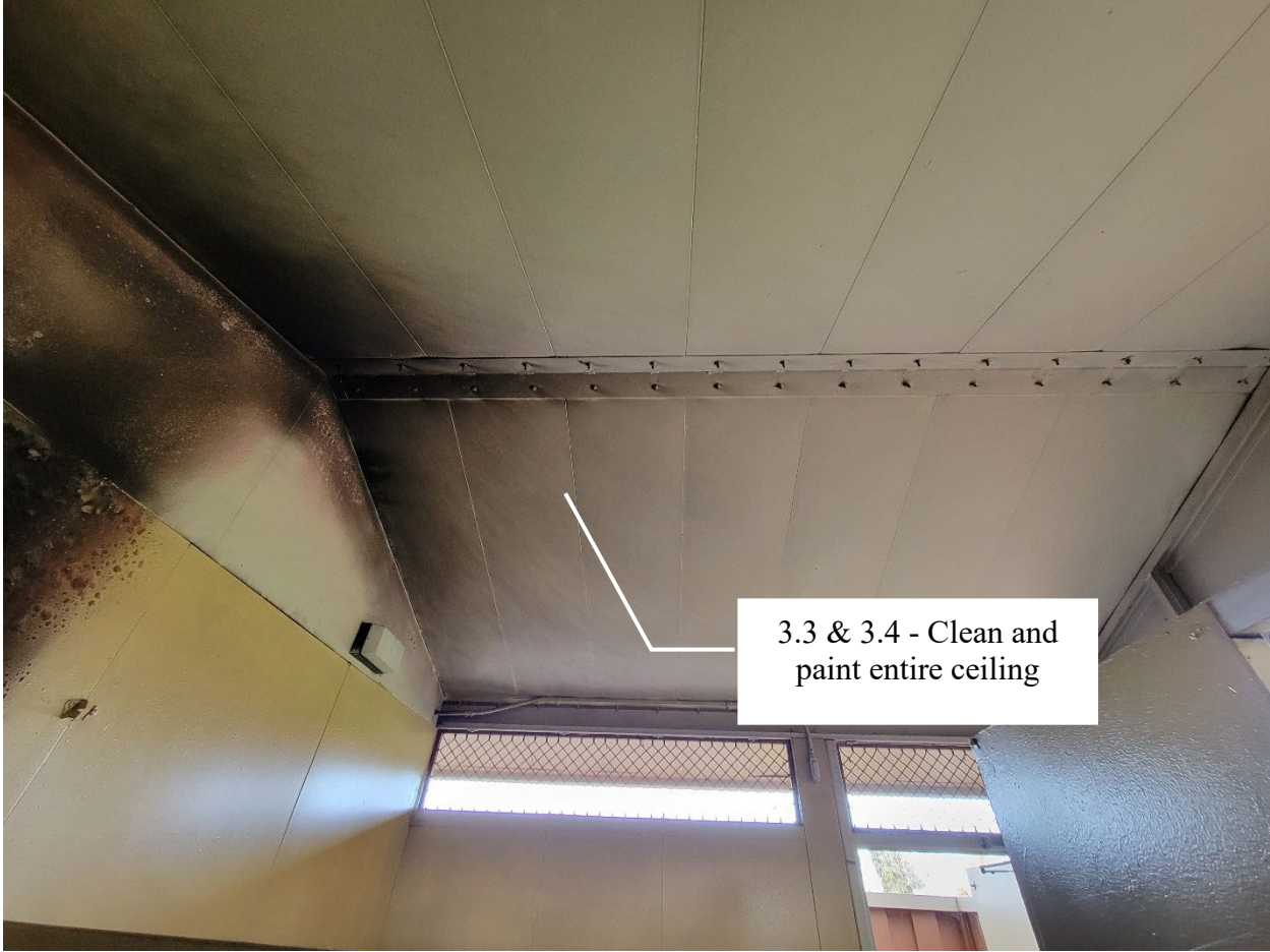
Figure 18 Harrington Men's Restroom Ceiling 1
