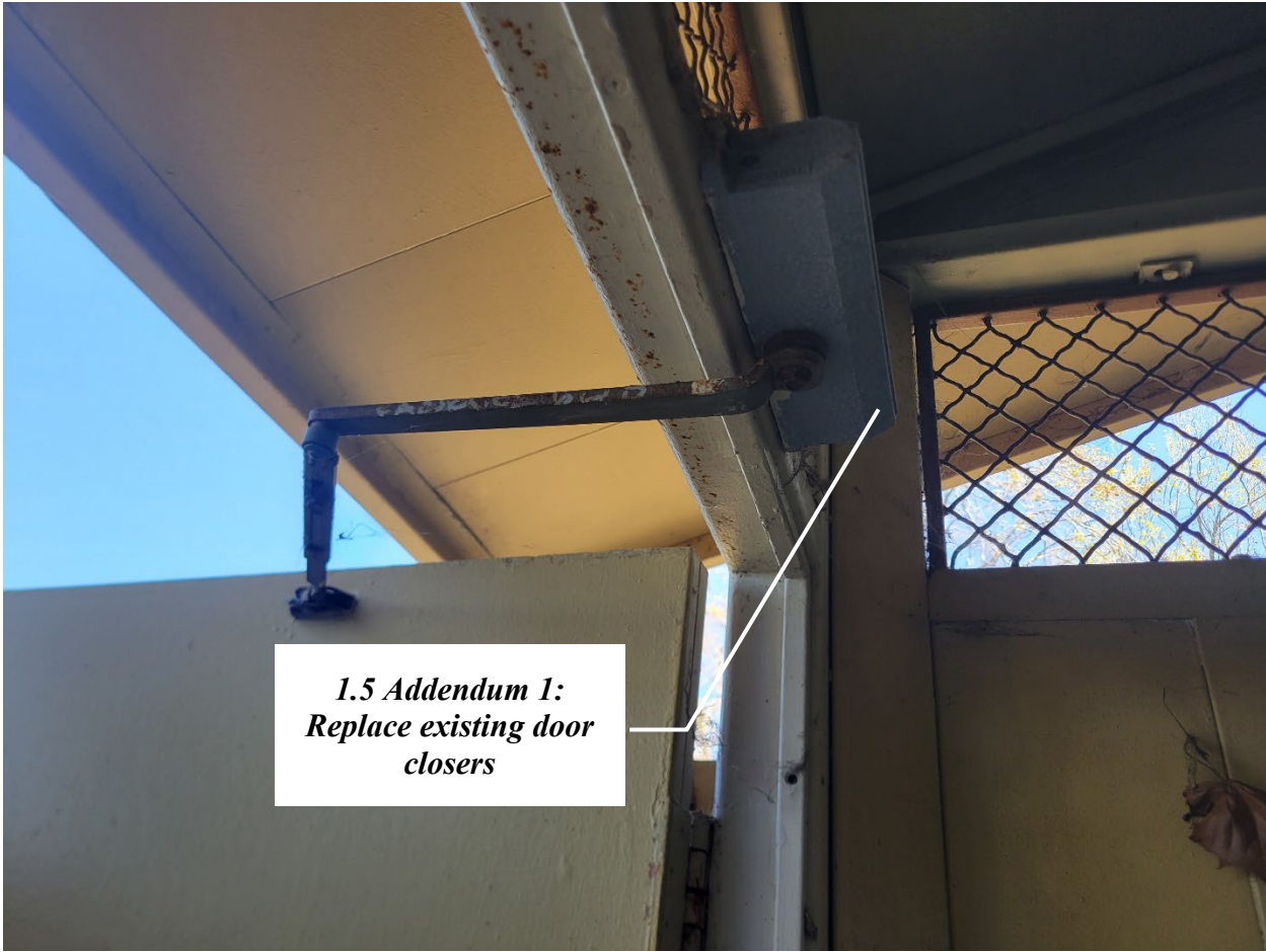
Figure 22 Addendum 1: Existing Restroom Door Closer
