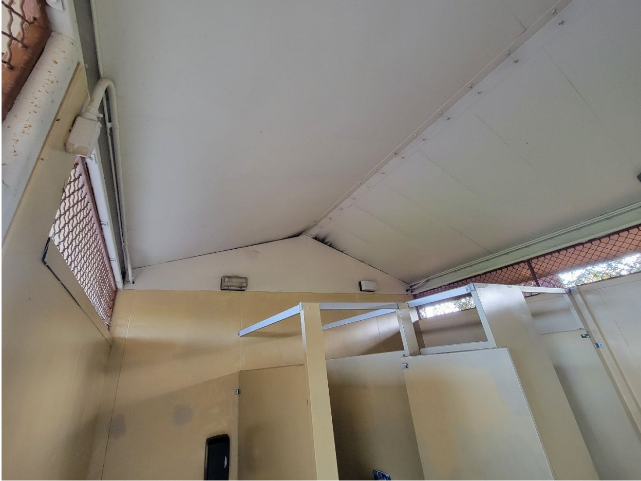
Figure 26 Harrington Women's Restroom Ceiling
