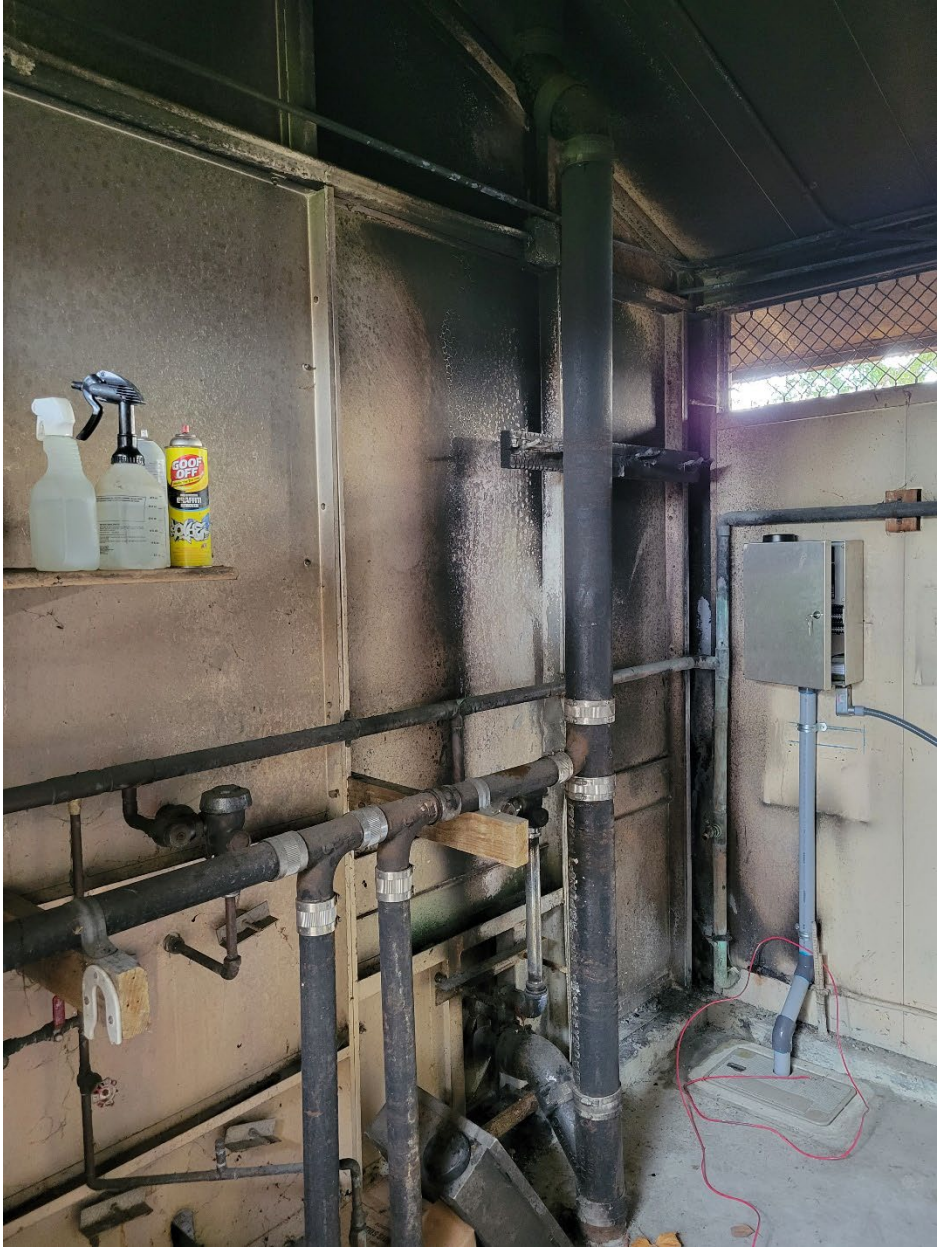
Figure 4 Harrington Utility Closet 2
