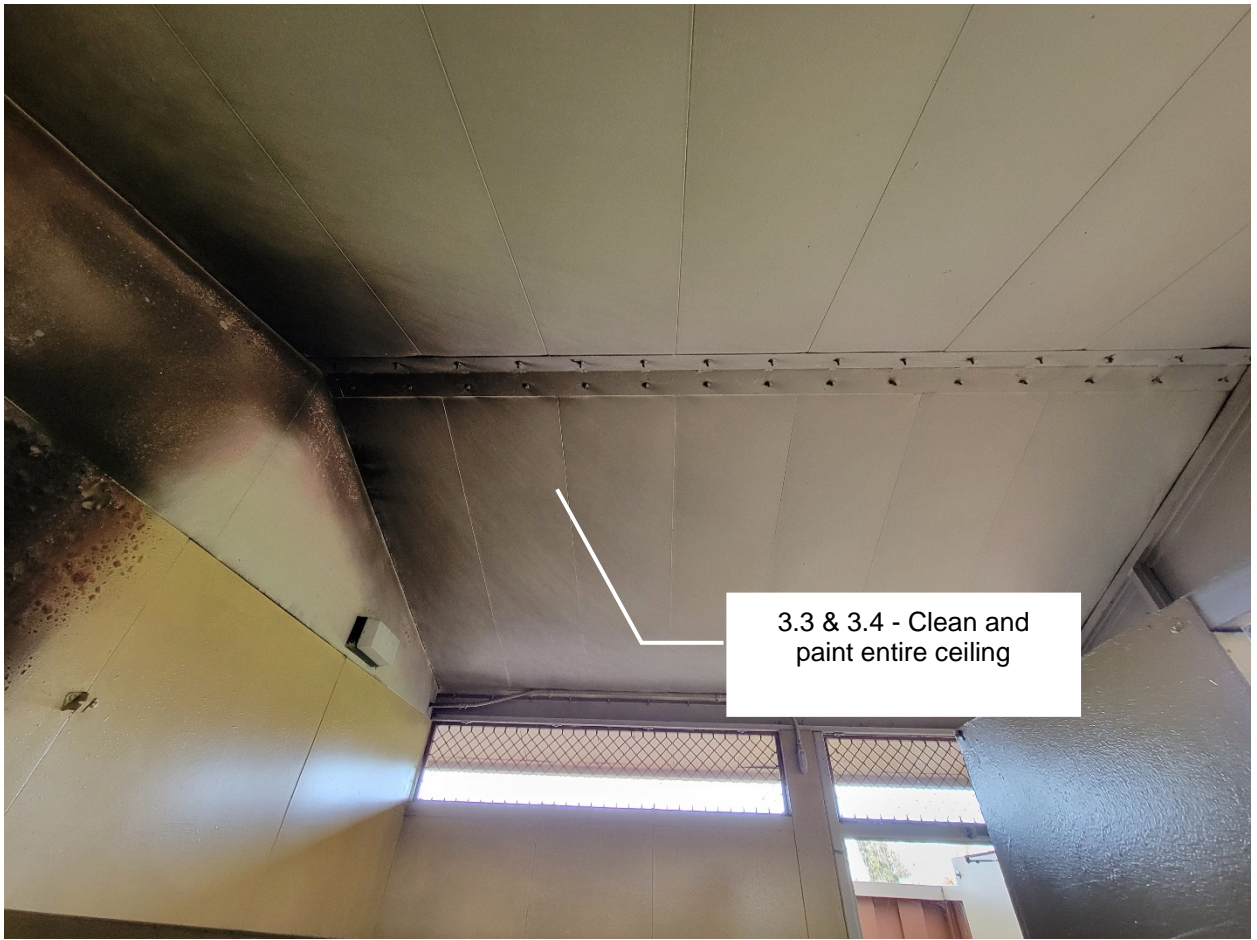
Figure 15 Harrington Men's Restroom Ceiling 1
