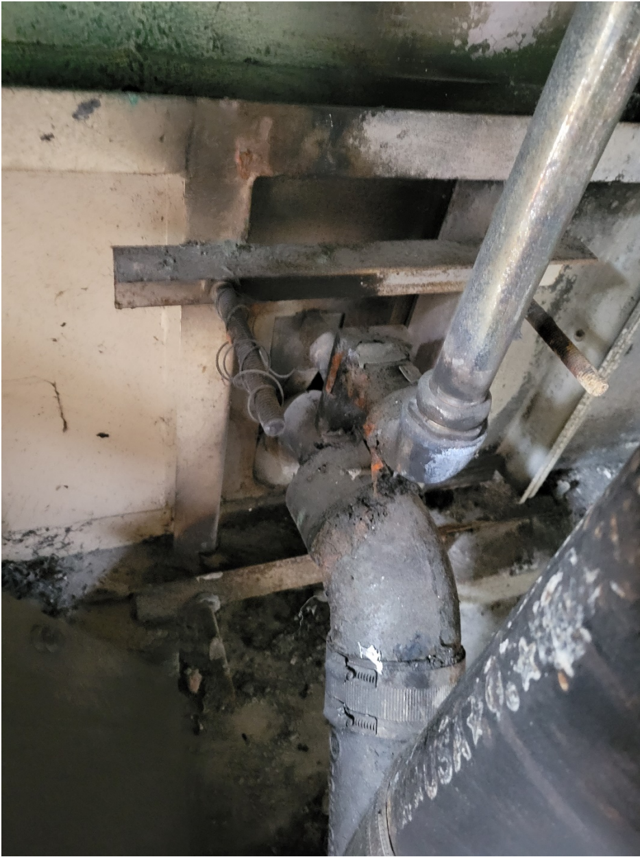
Figure 7 Harrington Utility Closet Plumbing 1
