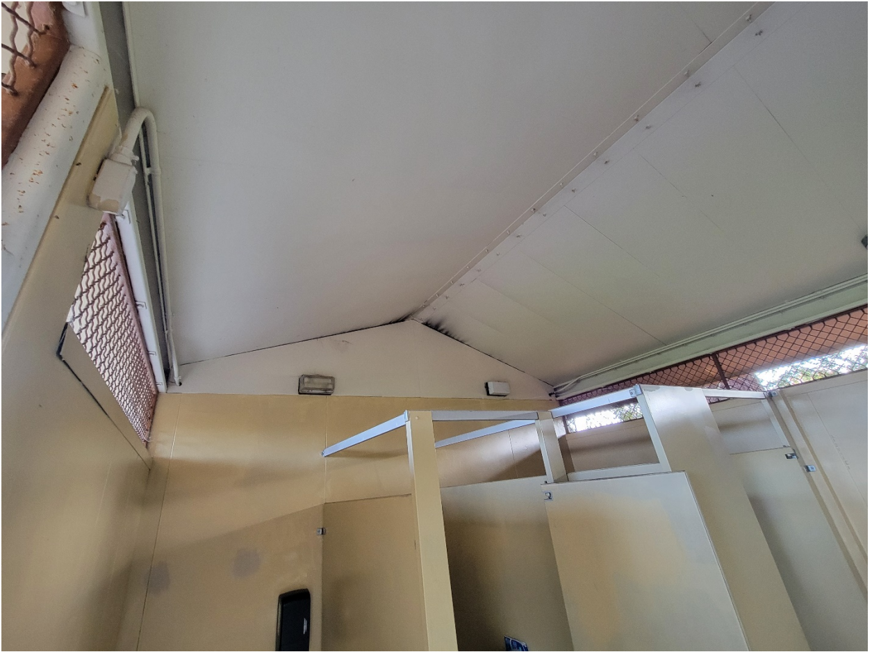
Figure 19 Harrington Women's Restroom Ceiling
