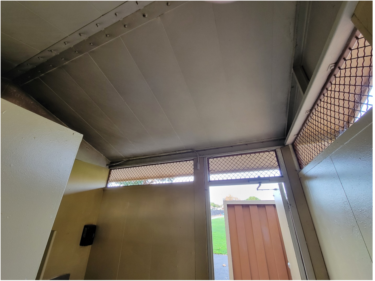
Figure 17 Harrington Men's Restroom Ceiling 2
