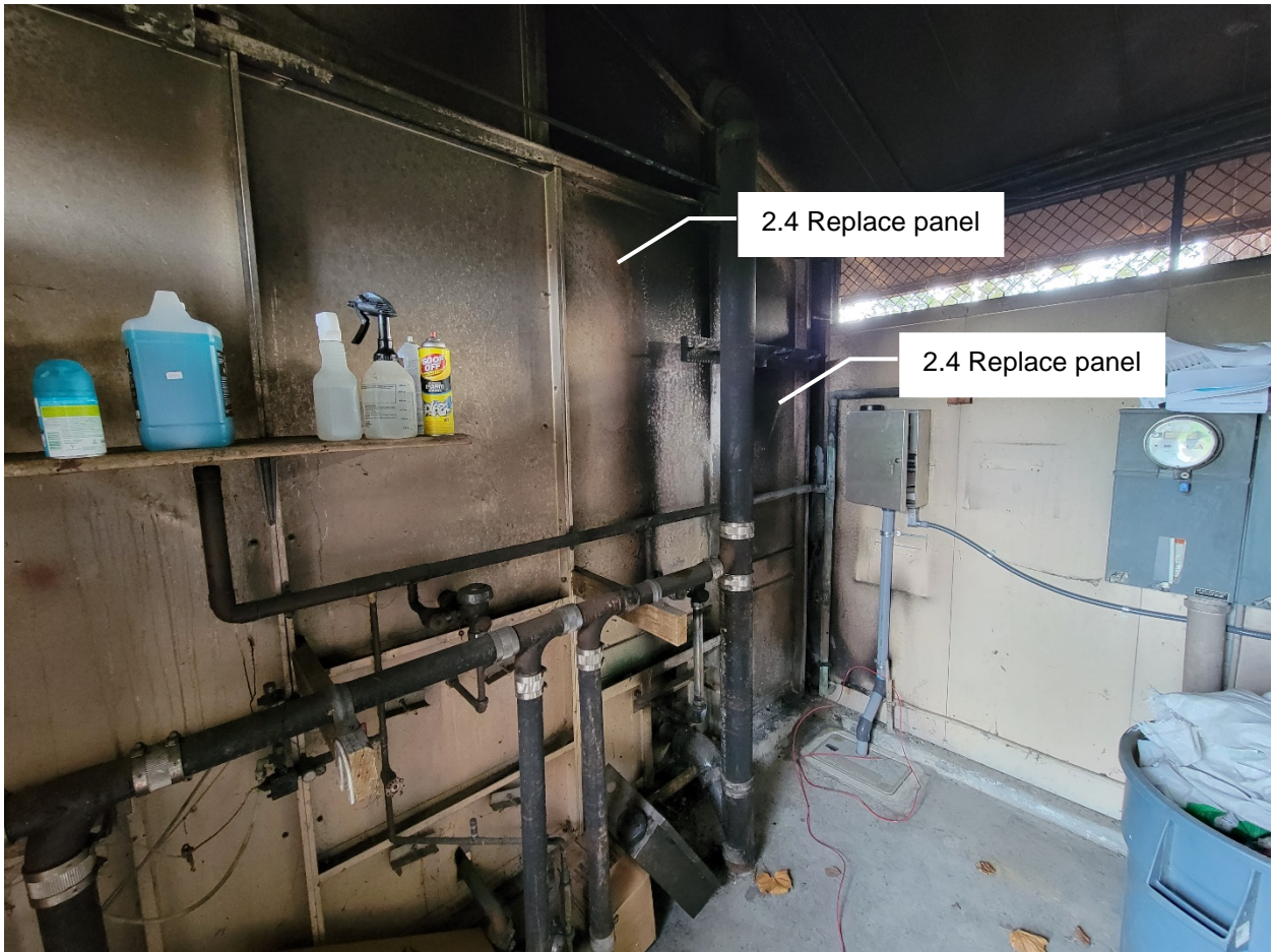
Figure 3 Harrington Utility Closet 1
