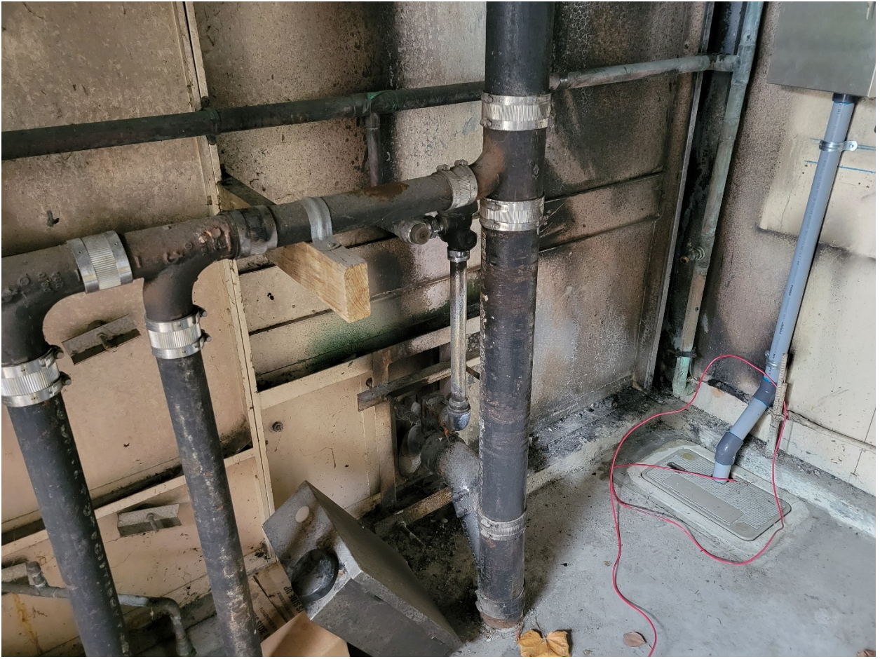
Figure 9 Harrington Utility Closet Plumbing 3
