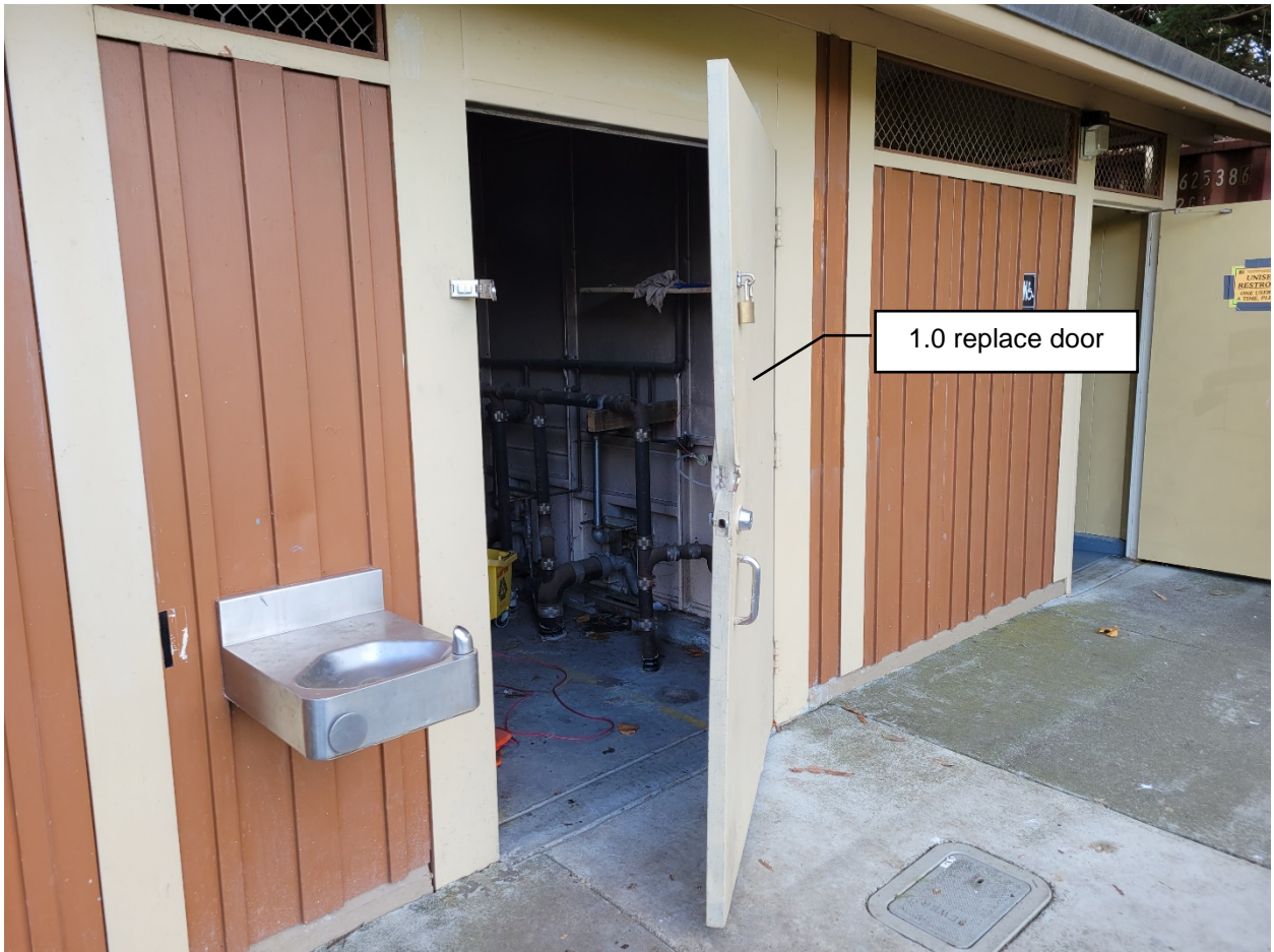
Figure 2 Harrington Utility Closet Door
