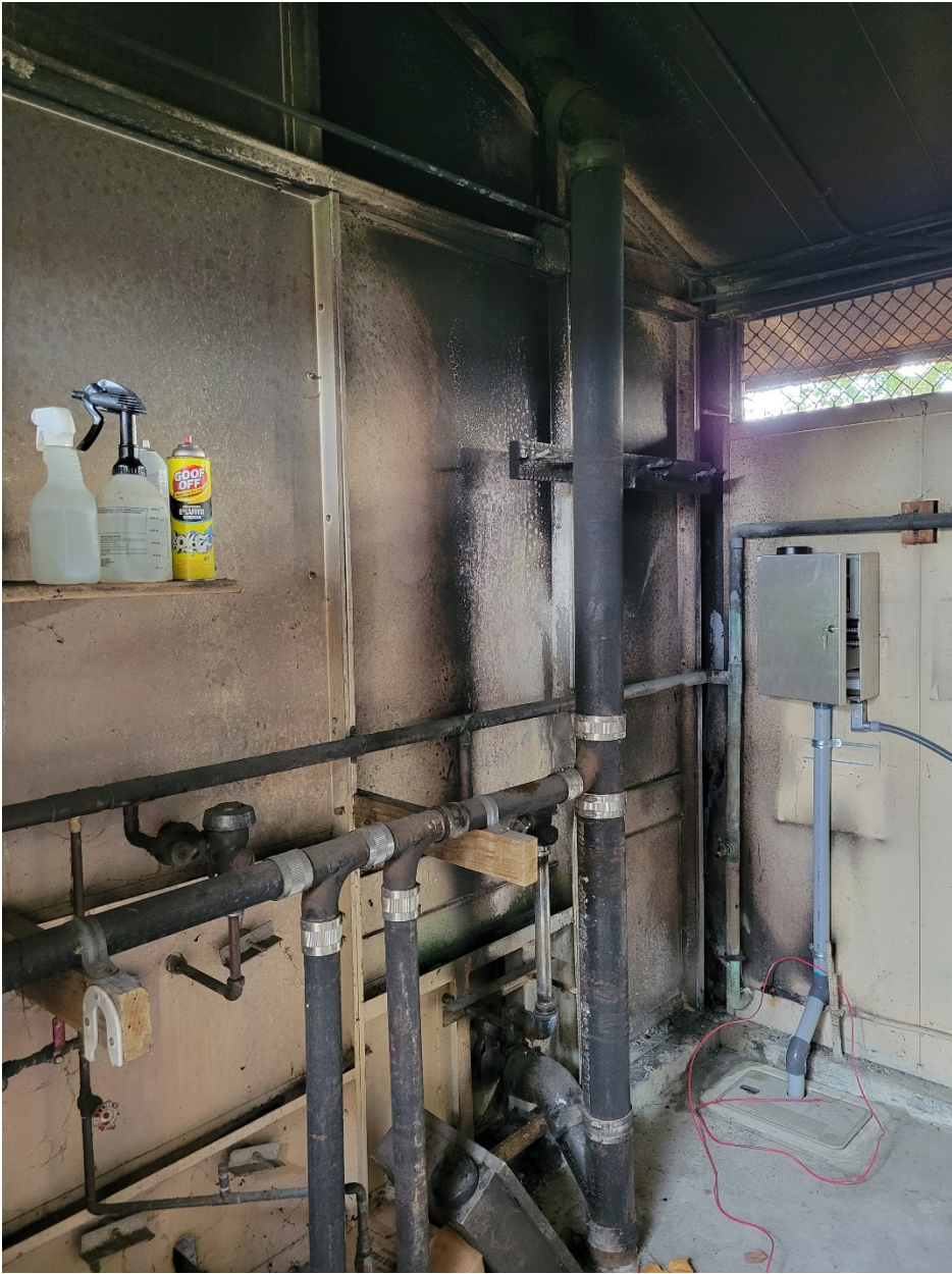
Figure 4 Harrington Utility Closet 2
