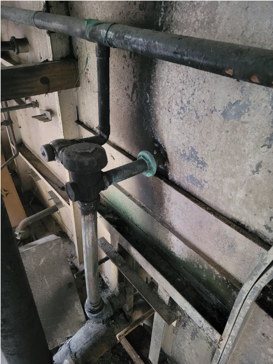
Figure 8 Harrington Utility Closet Plumbing 2
